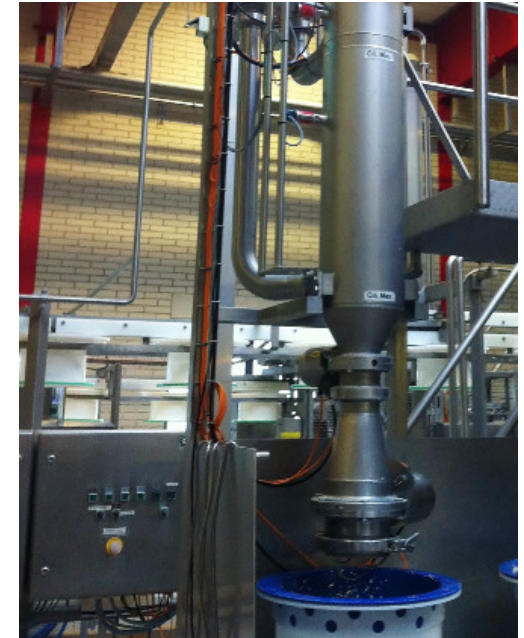
Modified Auto-line XL filter in the manufacturing of dairy products.
